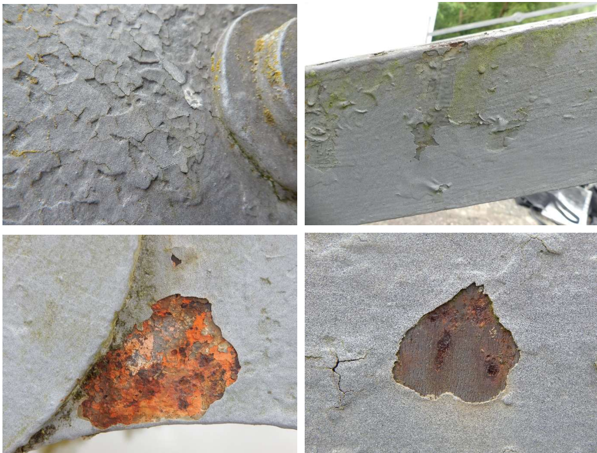
Figure 6 – Defect of painting system – typical examples
