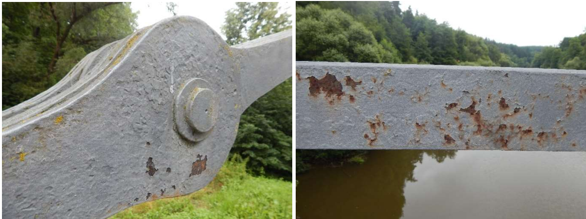
Figure 3 – Wrought iron parts (left - chain pin, right – chain link)
