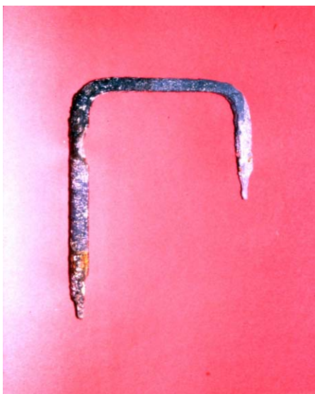
Figure 5. Corroded rebar from a 4 years old building in hot and salty environment
