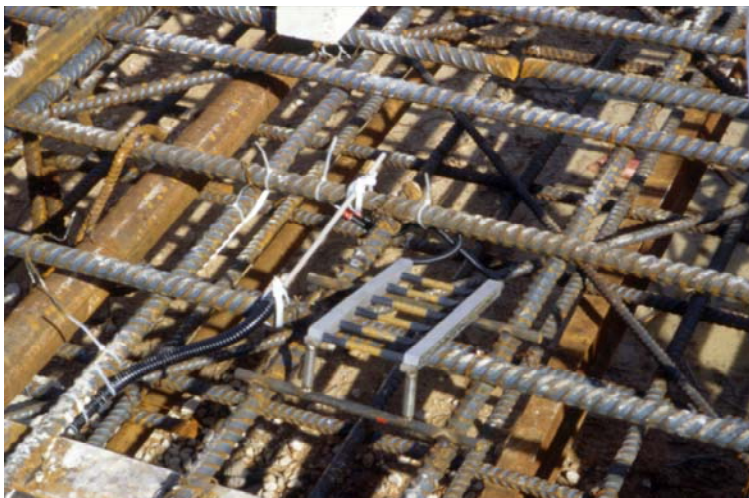
Figure 13. Sensors installed in a concrete structure to monitor the corrosion risk for the reinforcement
