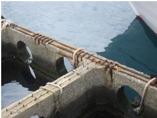
Figure 1. Example for chloride induced reinforcement corrosion in concrete exposed to seawater
