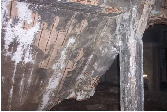
Figure 3. Corrosion of the reinforcement of an old concrete structure caused by insufficient concrete cover
