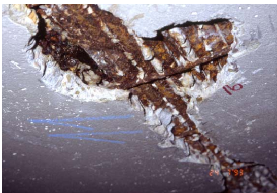
Figure 4. Corrosion of the reinforcement caused by local bad compaction of the concrete
