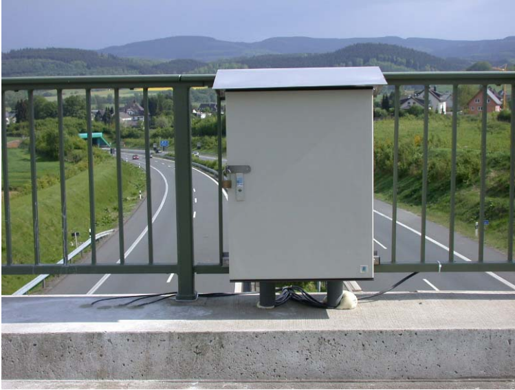
Figure 14. Measuring unit of exposure tests at a highway in Germany within the splashwater zone
