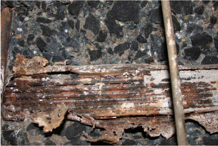
Figure 12: Corroding prestressing steels after opening of the duct
