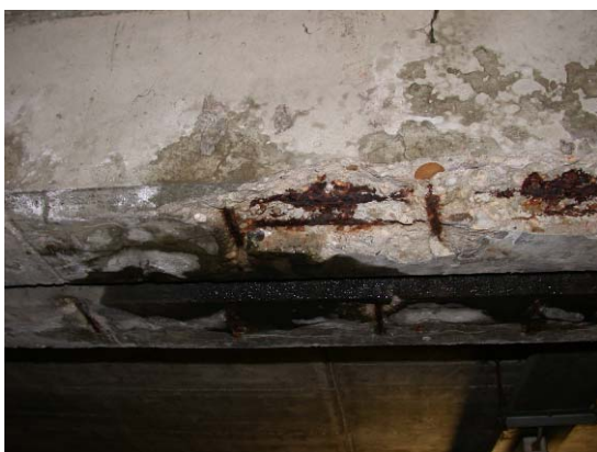
Figure 2. Example for chloride induced corrosion of the reinforcement exposed to deicing salts within a leaking joint of a parking garage
