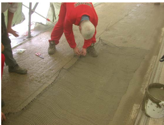
Figure 9. Cathodic protection by an impressed current using a carbon mesh anode in a special mortar
